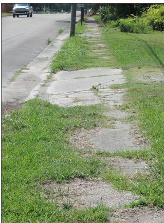
Bridgeton is already working to repair and replace many of the sidewalks that are in poor condition, like this one on B Street near Academy St.
